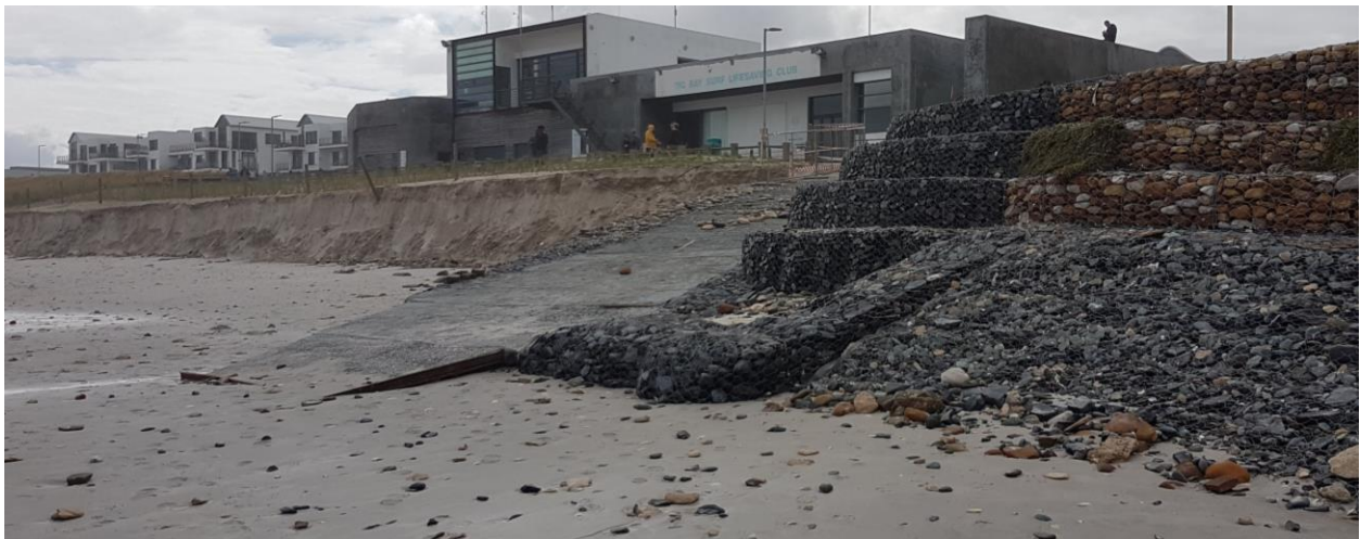
Figure 1-1: Eroded beach in front of the lifesaving building (April 2018).
